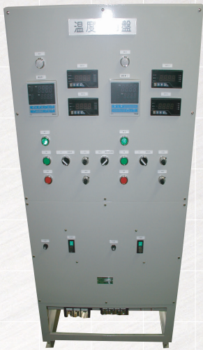
各種温度制御盤 Various Temperature Control Panel
